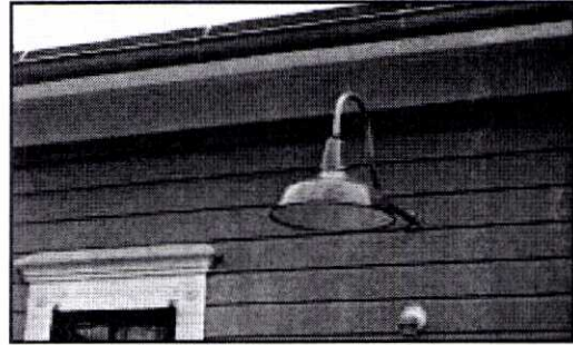
Appropriately shielded fixture with motion sensor.
