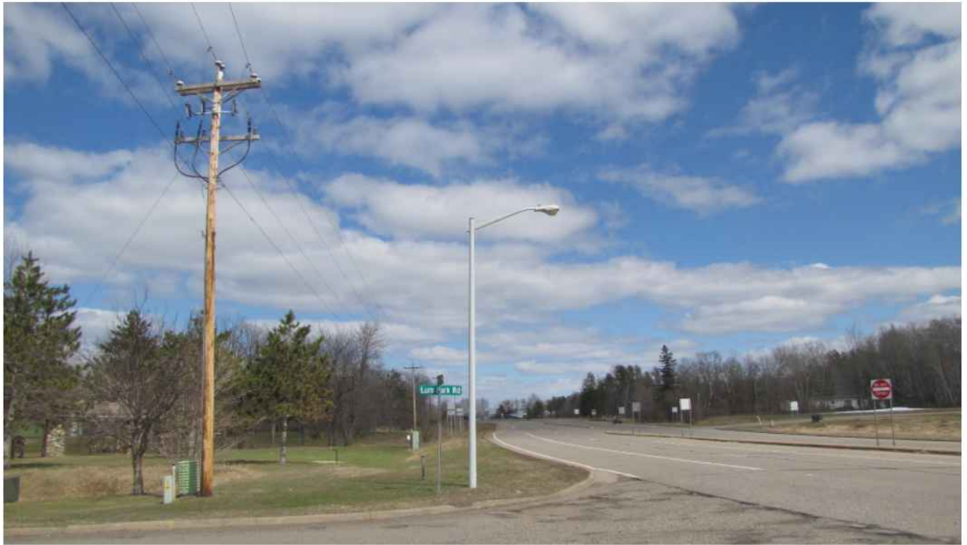
VIEW OF OVERHEAD POWER ALONG NORTH SIDE OF HIGHWAY 210 FROM NORTH SHOULDER LOOKING EAST
