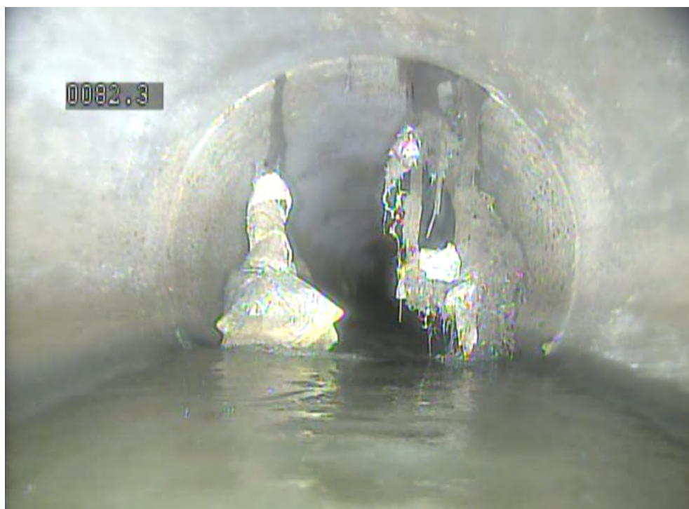
Image 2: Significant Root Intrusion, Pipe 09-08
