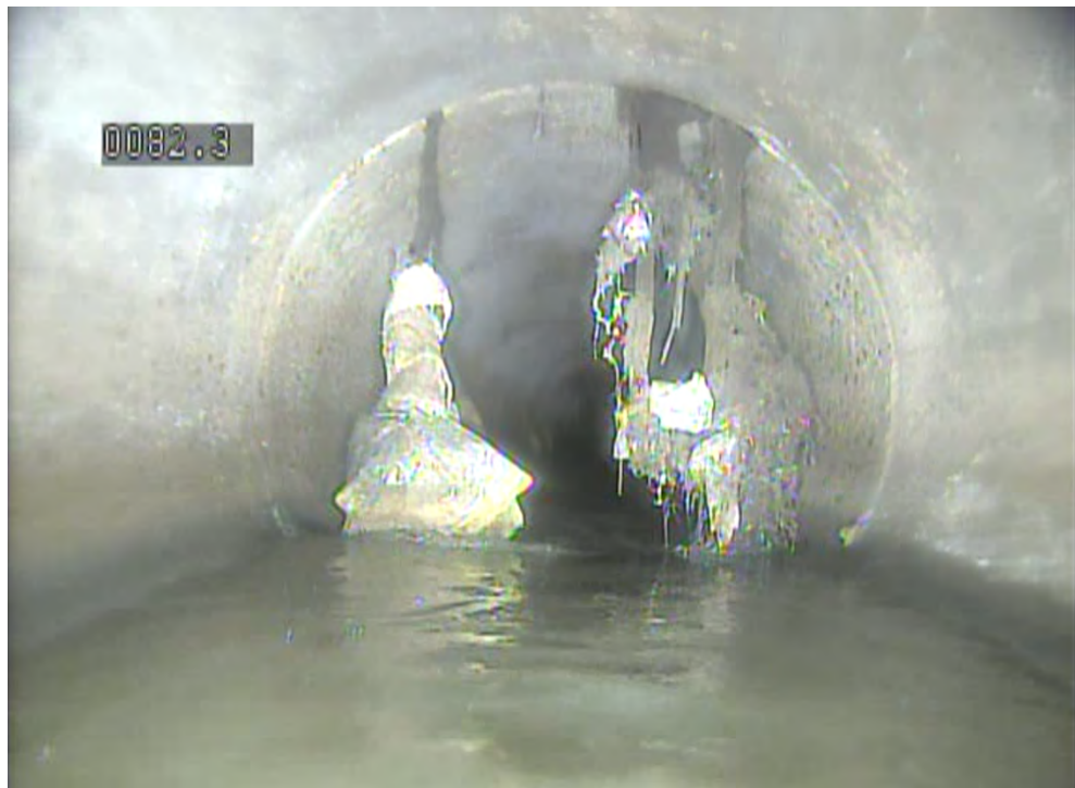
Image 2: Significant Root Intrusion, Pipe 09-08
