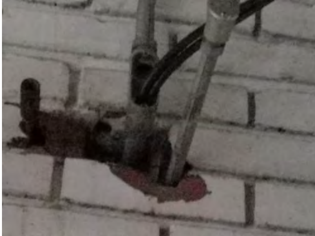
Outlet Next to Panel missing a Screw
