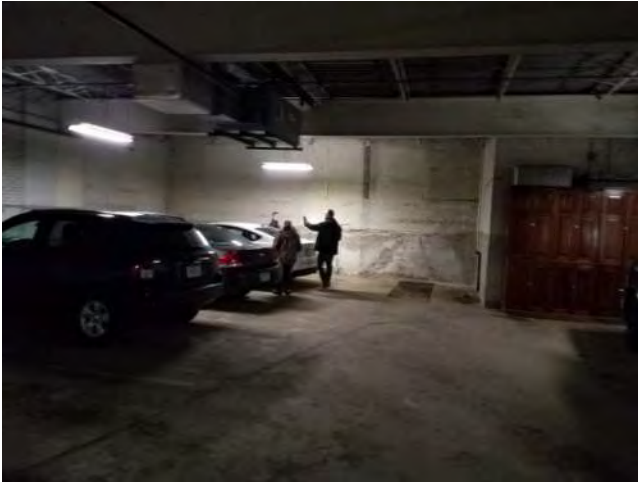
Old Cloth Covered Cables Need to be removed
