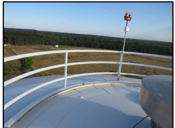
Obstruction Lights at Top
