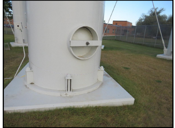
Tank Riser at Base
