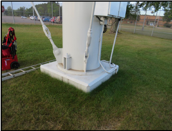
Tank Leg at Base
