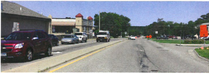
CSAH 20 (NW 4 th Street) is in need of repair and capacity expansions at the TH 210 intersection.
