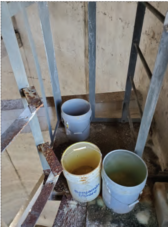
12) Top of stairs. Note rust and evidence of water infiltration, 2020
