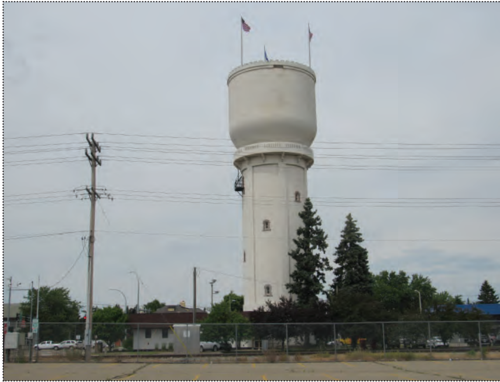
4) Looking north. Note delamination just below crenelations
