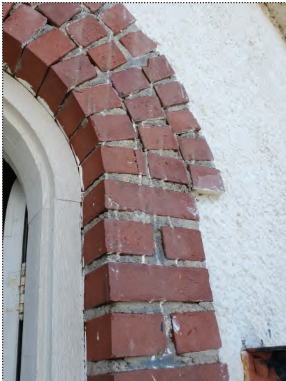
16) Typical mortar condition at brick surrounds, 2020
