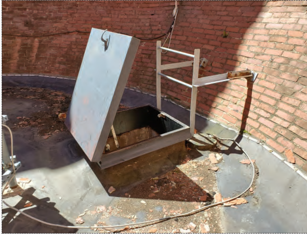
9) Hatch at base of bowl. Note masonry debris, 2020
