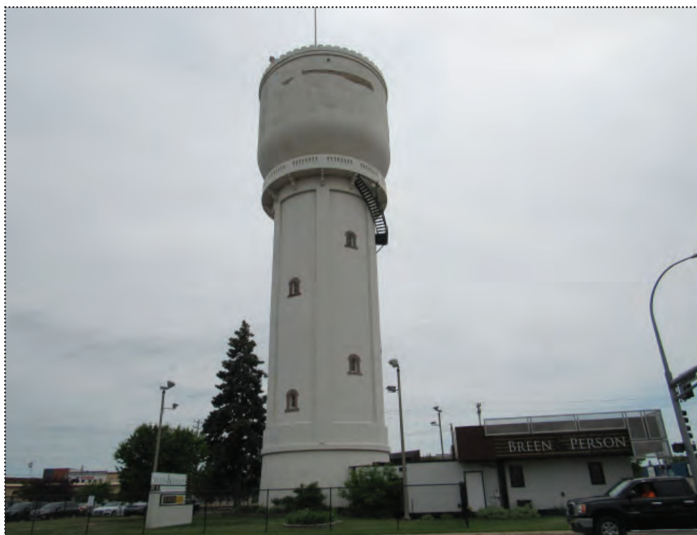
3) Looking south. Note delamination near top of bowl
