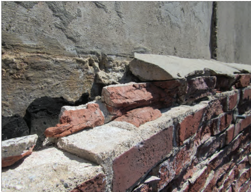
10) Deterioration at top of brick liner. Note bituminous waterproofing behind, 2020
