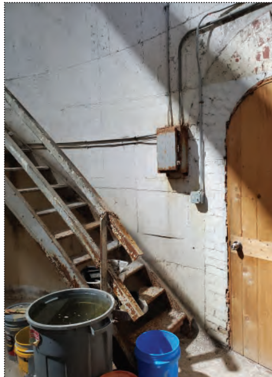
13) Bottom of stairs. Note rust and evidence of water infiltration, 2020
