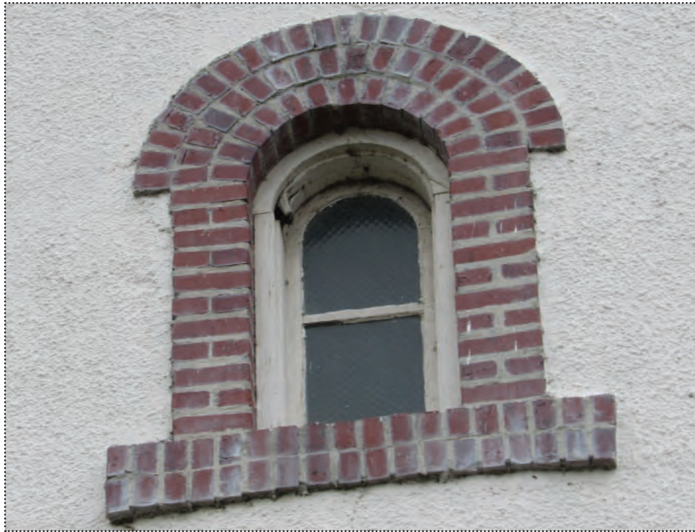
18) Window 10. Damage at this window appears to be the most significant of all windows, 2020
